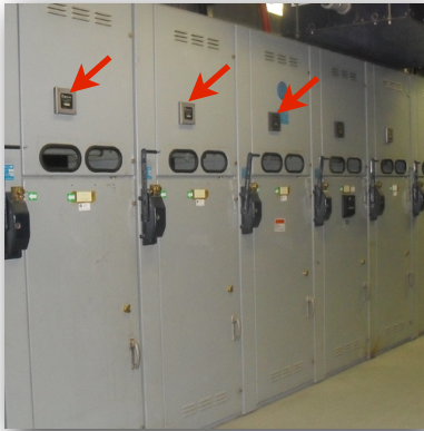
Fig. 1: IR Windows mounted in switchgear
